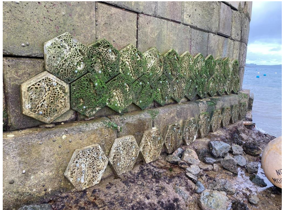
Fig 8. Sea wall tiles attached to a harbour wall in the inner harbour.
